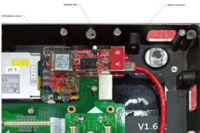
Typical installation of an indoor node
